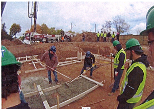
Students poured the foundation at the Raise Me Up house in Welland last fall.
